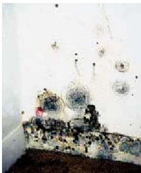
From EPA Mold Remediation in Schools and Commercial Buildings Guide
