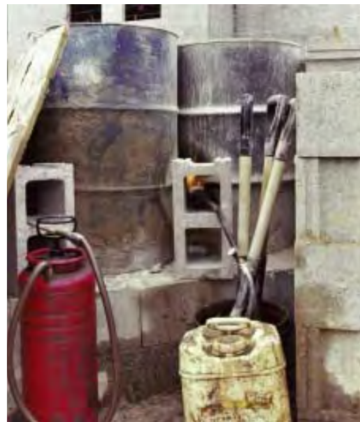
Fig. 5-4 A propane torch is used to heat the water that will be used in mortar mixing. (IMG12507)
