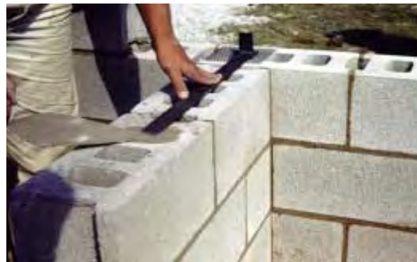
Fig. 4-47 Steel tiebar provides lateral support to wall at back in photo. (IMG4019)
