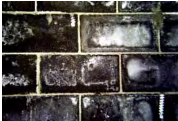
Figure 2-10 A severe case of efflorescence. (IMG15607)
