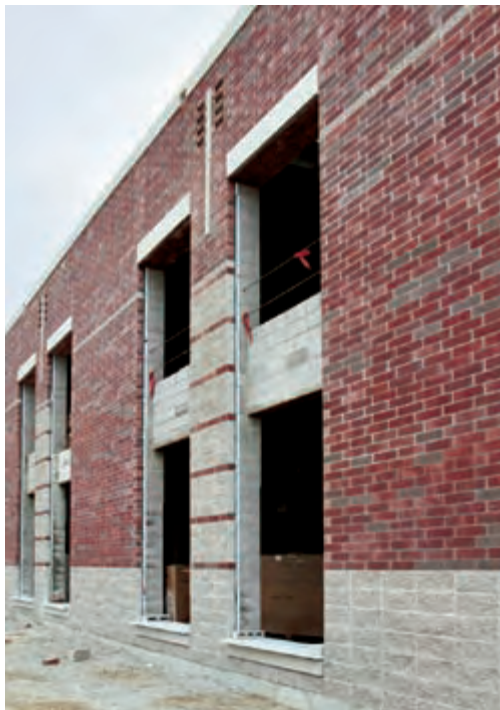
Fig. 4-8a A reinforced concrete masonry wall veneered with brick. The collar joint is not filled with mortar. (IMG24954)
