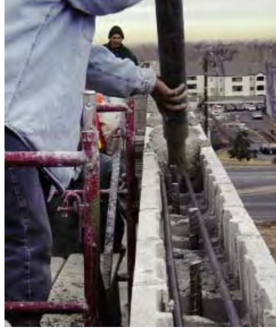
Fig. 6-48 Horizontal reinforcing bars positioned in a bond beam that will be solidly grouted. (IMG24196)
