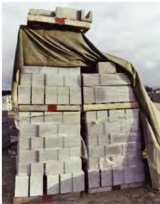
Fig. 5-3 Concrete masonry units covered with canvas or plastic tarpaulins to keep the block dry. (IMG12505)
